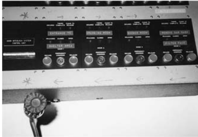
Control panel that would have been used to secure the nuclear-proof command post, RAF Bentwaters (1999) © Georgina Bruni
