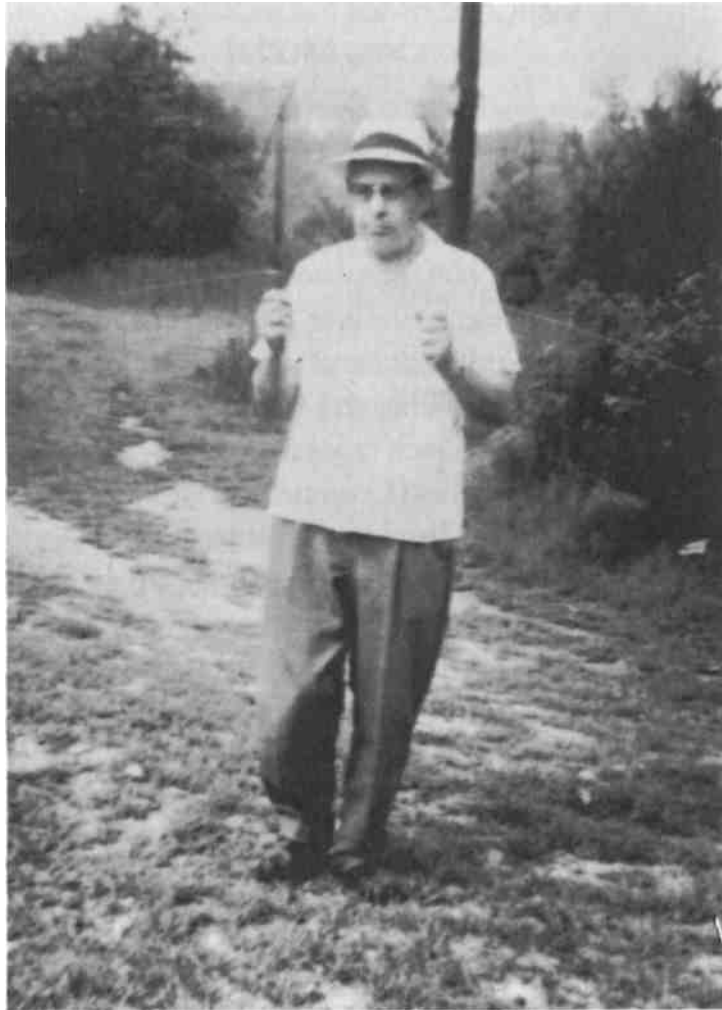
Figure 2-1: Employee of the Milford, Connecticut, water company using detector rods to locate city's water mains. Employee did not wish to be identified nor would he permit a second photo session.
