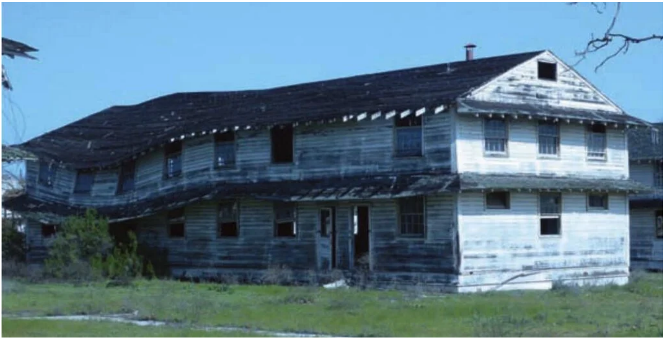
One of the hundreds of condemned buildings at Camp Roberts, many of which contain lead, asbestos, and other contaminants. Source: Wikimedia
