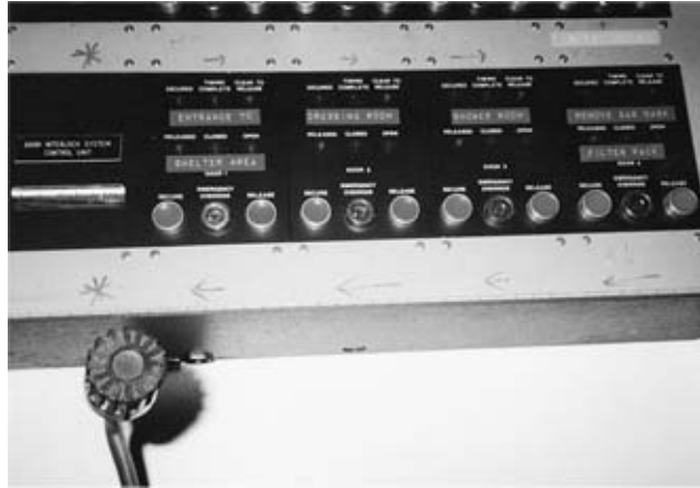
Control panel that would have been used to secure the nuclear-proof command post, RAF Bentwaters (1999) © Georgina Bruni
